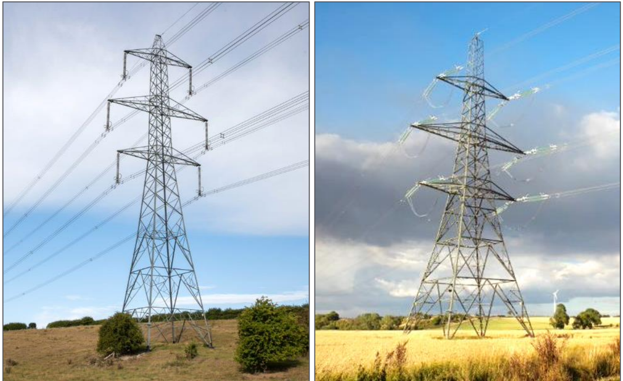
Image 4.2: Suspension Pylon (left) and Angle Pylon (right)
