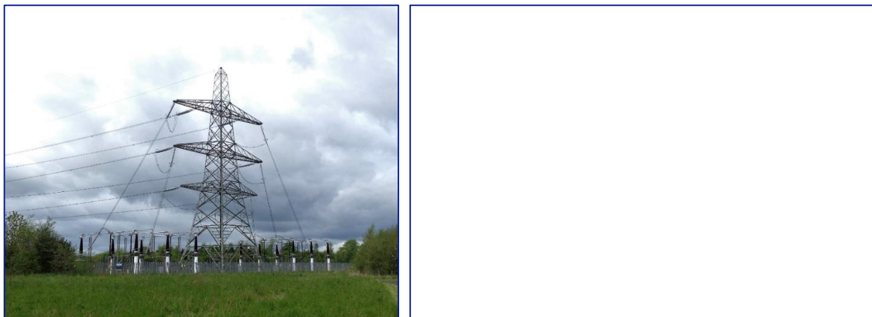
Image 4.5: Example 400 kV sealing end compound
